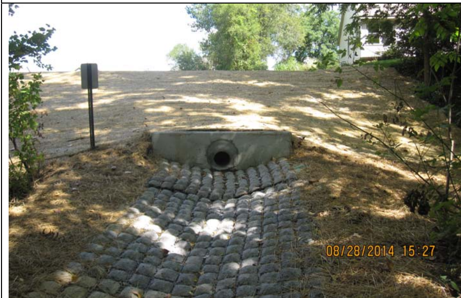
Photo #7: Installed new ditch below outlet culvert. Placed flex-a-mat material across the ditch from pipe to the stream channel.
