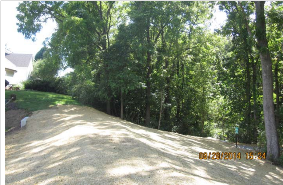
Photo #5: Finished grading of dam's crest and outslope. Removed the tree stumps, debris, wire fencing, etc. Added clean soil fill.
