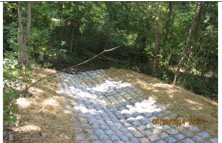
Photo #8: Installed new ditch below outlet culvert. Placed flex-a-mat material across the ditch from pipe to the stream channel.
